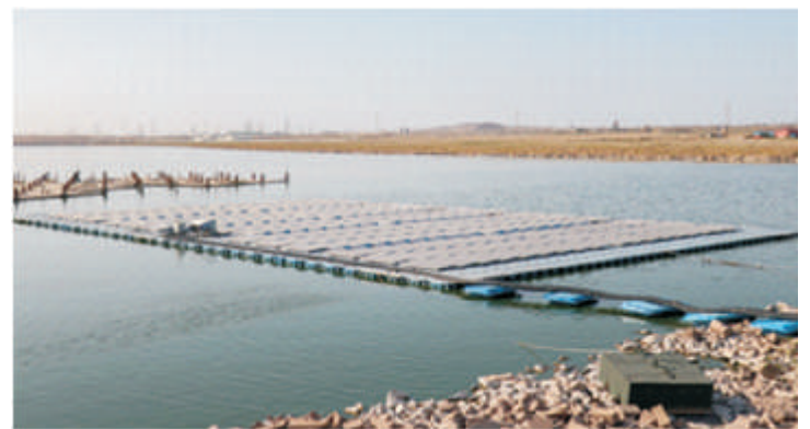
The floating solar power plant installed on the Lake Boyukshor in the suburbs of Azerbaijan's capital Baku / 1News.az
